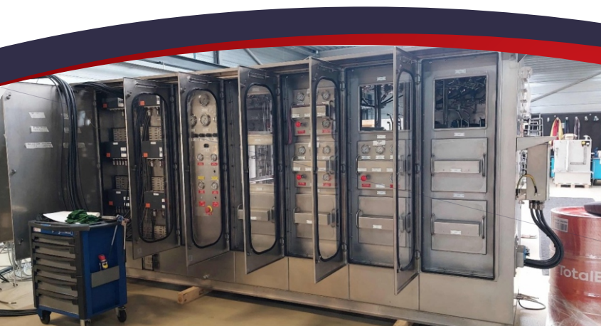
TOTAL WELLHEAD CONTROL PANEL & HYDROLIC UNIT
